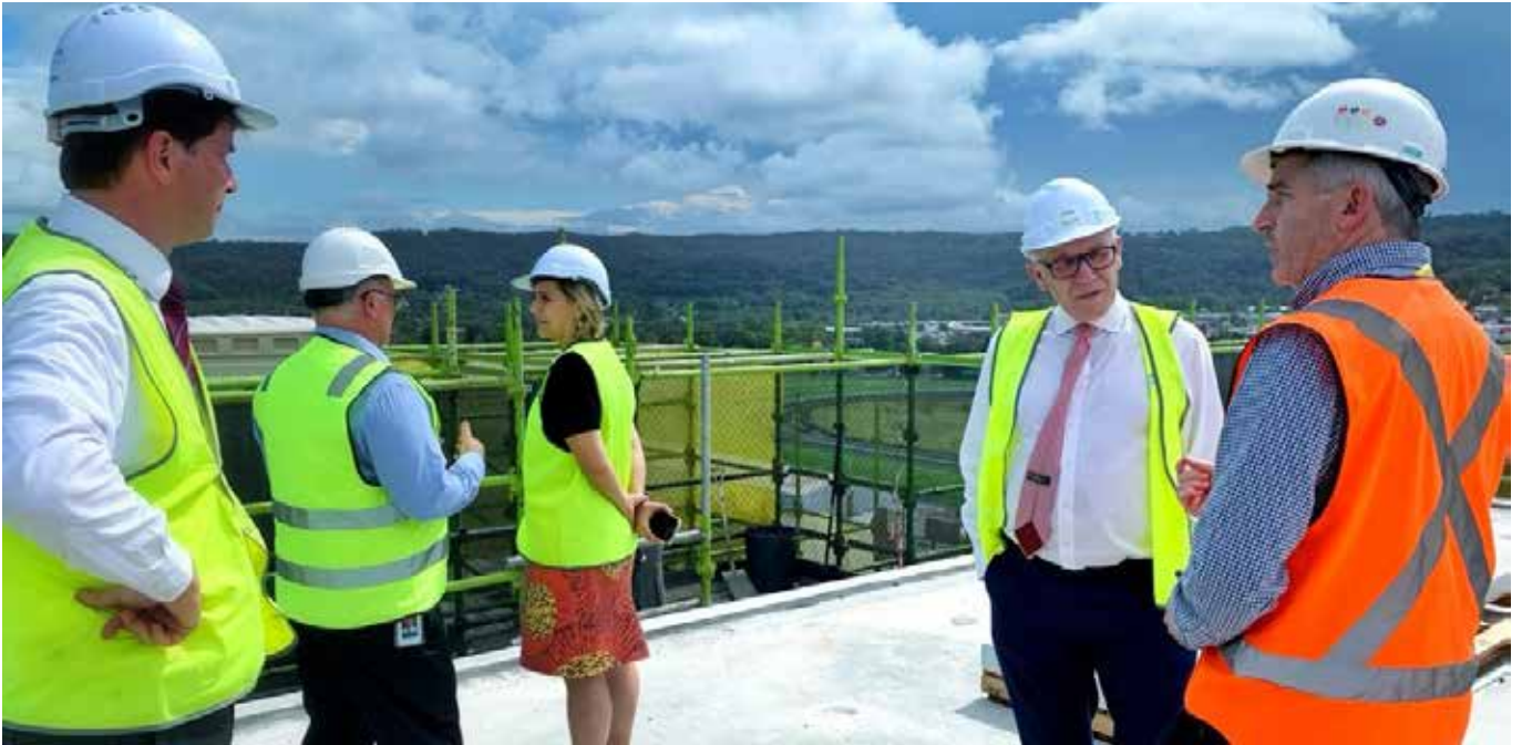
Inspecting a new construction project on the Central Coast in December with Finance and Small Business Minister Damien Tudehope
